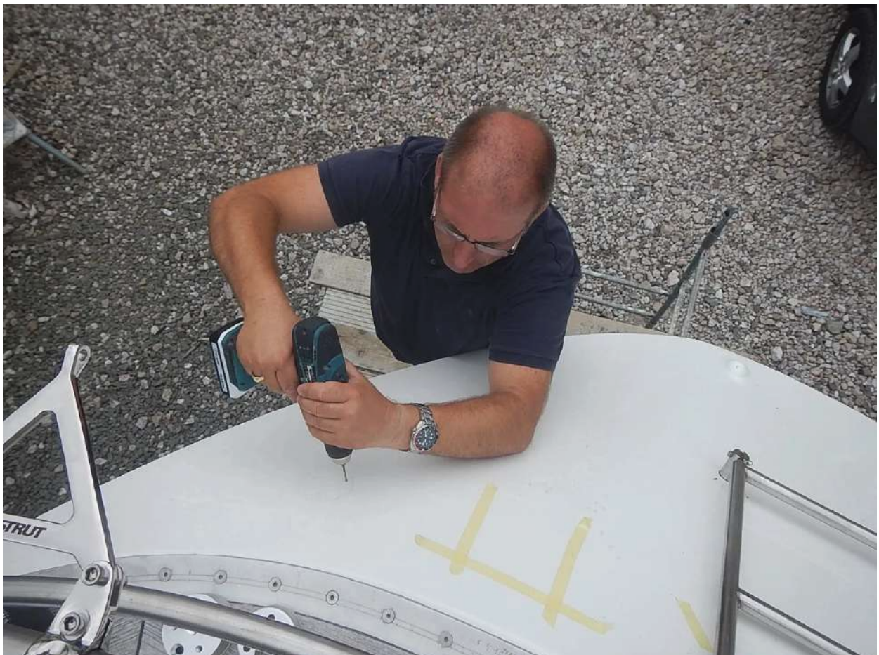
Drilling the base plate mounting holes in the transom which secure the bottom of the Radar pole in position. The masking tape marks an area on the transom which must not be drilled into.
